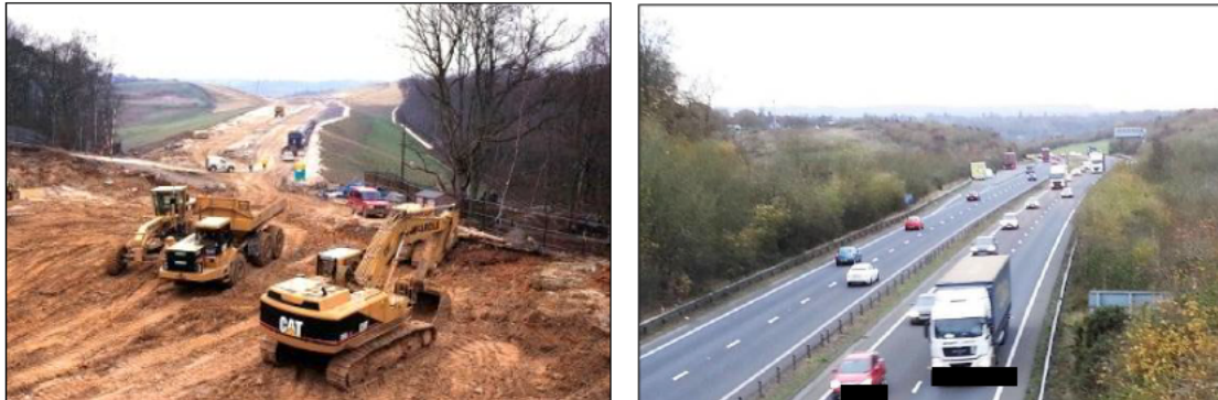
Figure 7.7: Excavation of cuttings for Newbury Bypass and a close-by vantage point in 2016
